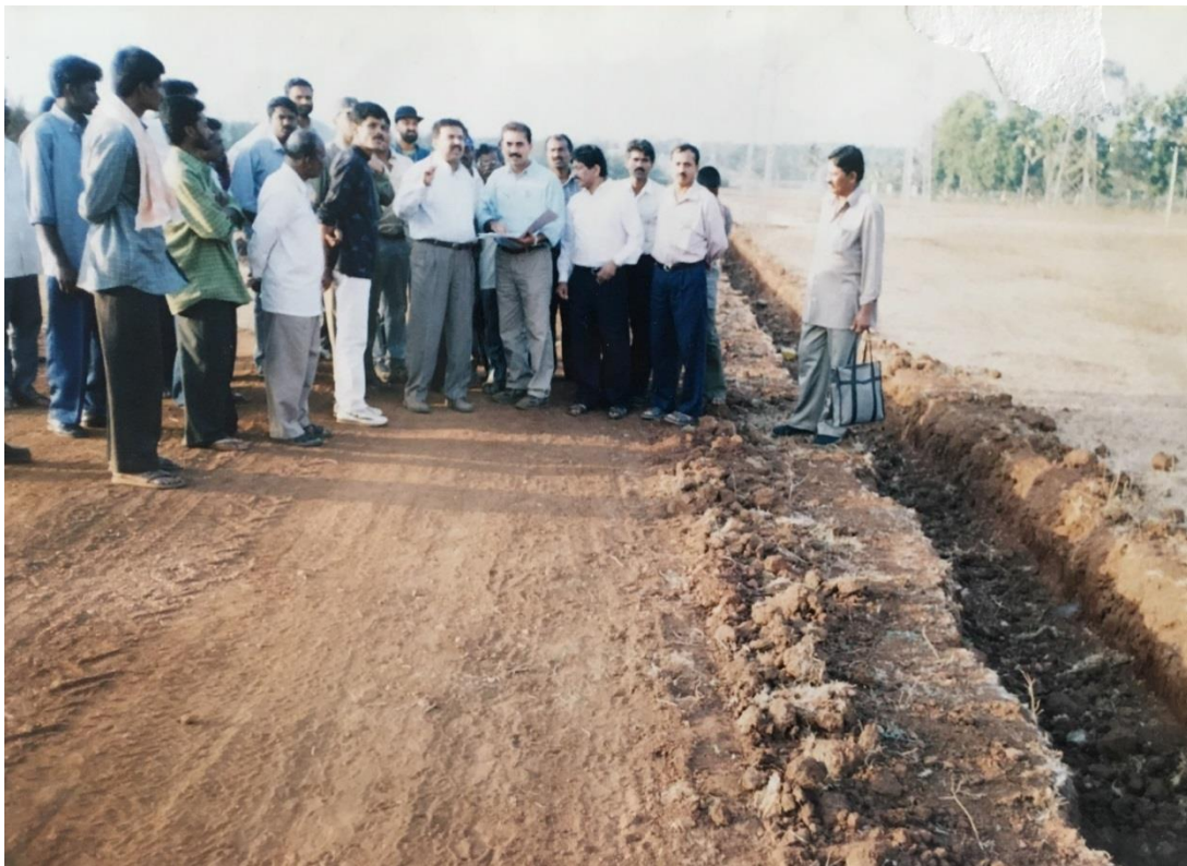
MC Halli site inspection by Gopalakrishne Gowda with the DCF and other officers during Bhadra relocation. Photo credit : DV Girish
